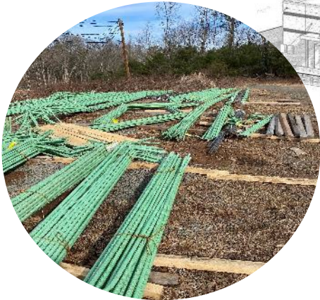
Hunt Water Treat Plant East Windsor
