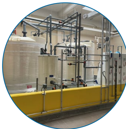
Mackenzie Water Treatment Clinton
